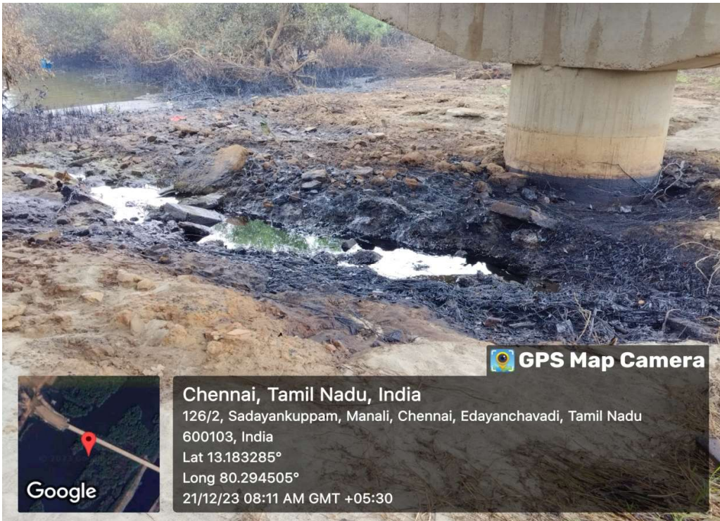
Figure 30: Oil contamination in Zone 8
