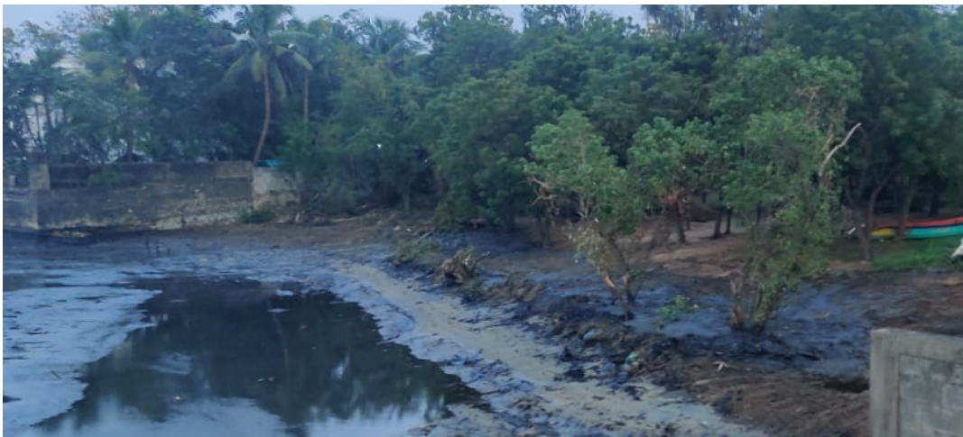
Figure 12: Earth moving machinery at the oil spill site
