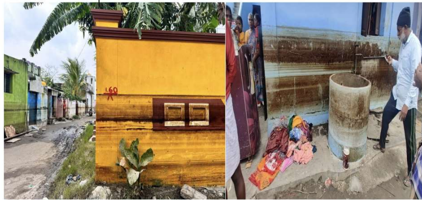
Figure 36: Oil stains seen on the walls of the residential buildings
